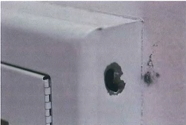
Fire extinguisher box
